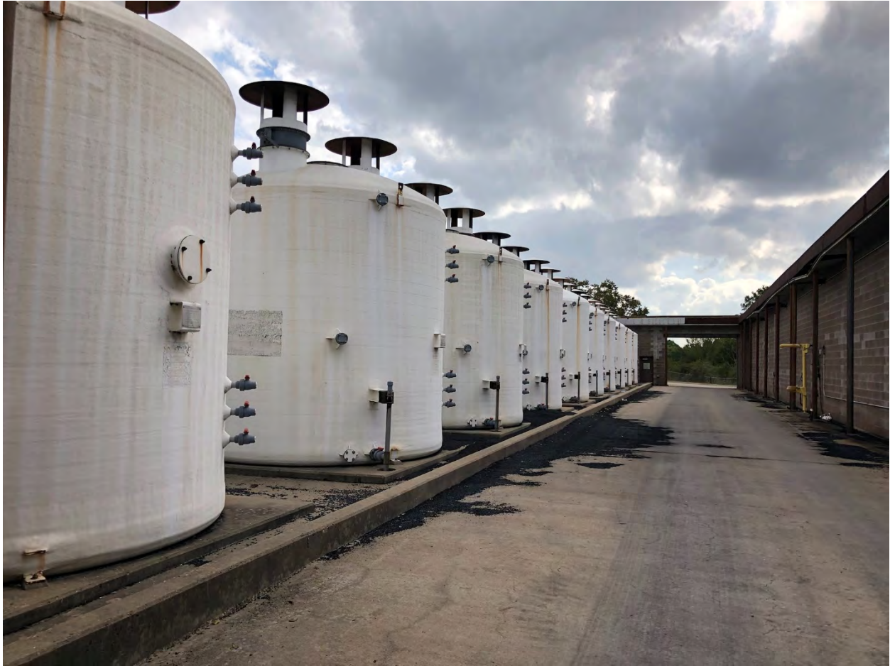
Figure J-12: Carbon Adsorption Odor Control Units
