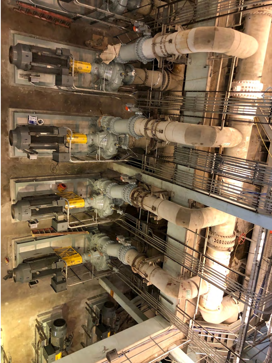
Figure J-5: Settled Wastewater Pumps in Operations Building
