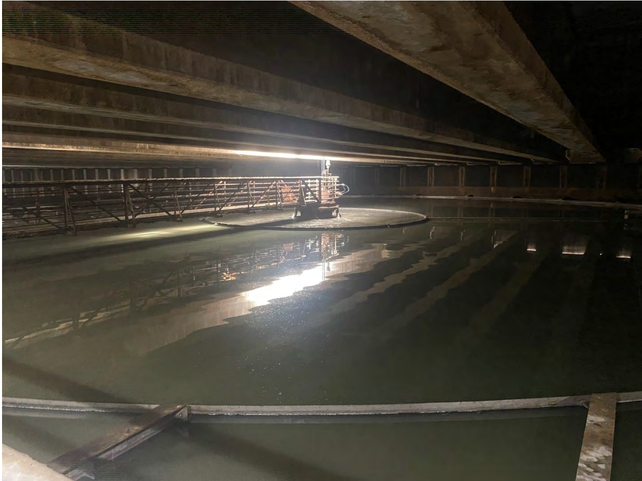
Figure J-3: Primary Clarifier in PTC 2
