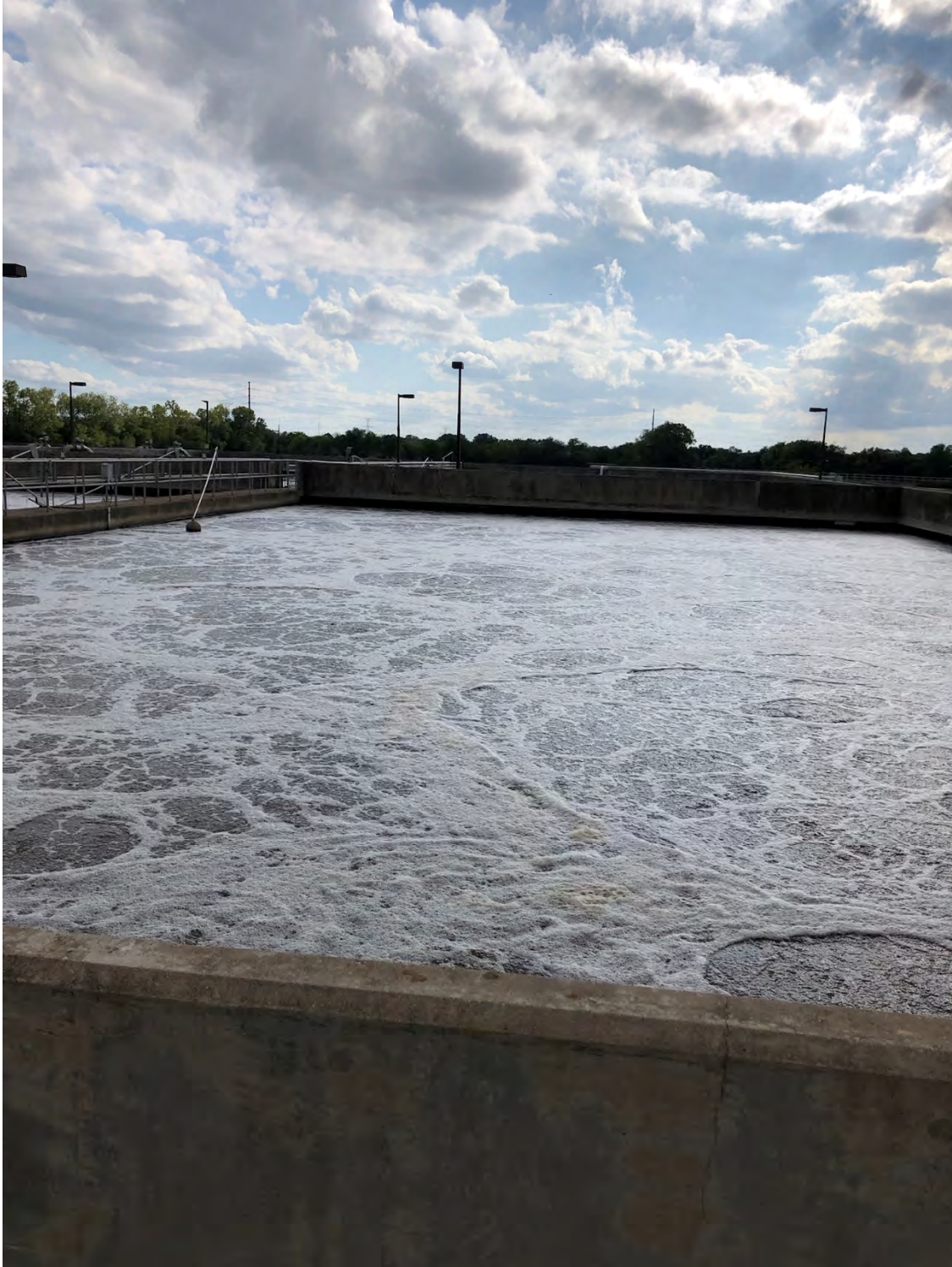
Figure J-6: Aeration Basin in ASC 1
