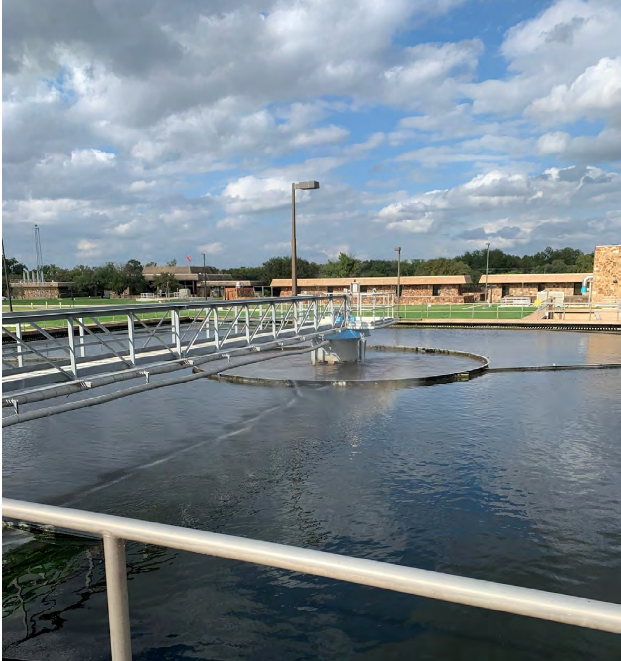
Figure J-8: Final Clarifier in ASC 1
