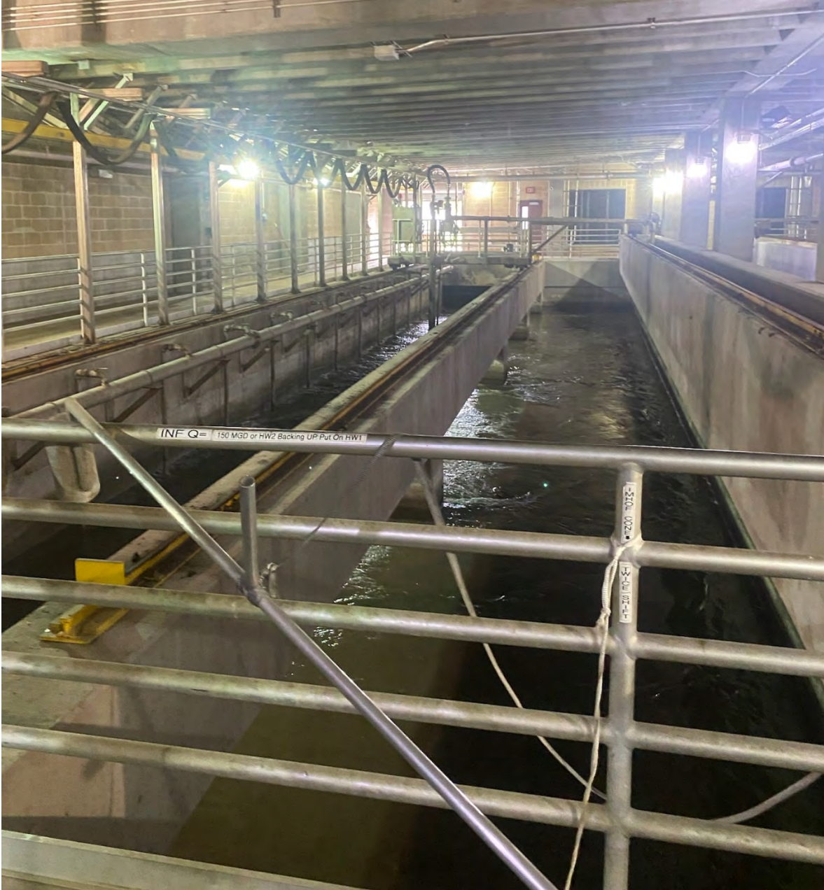
Figure J-2: Grit Chamber in HW 2
