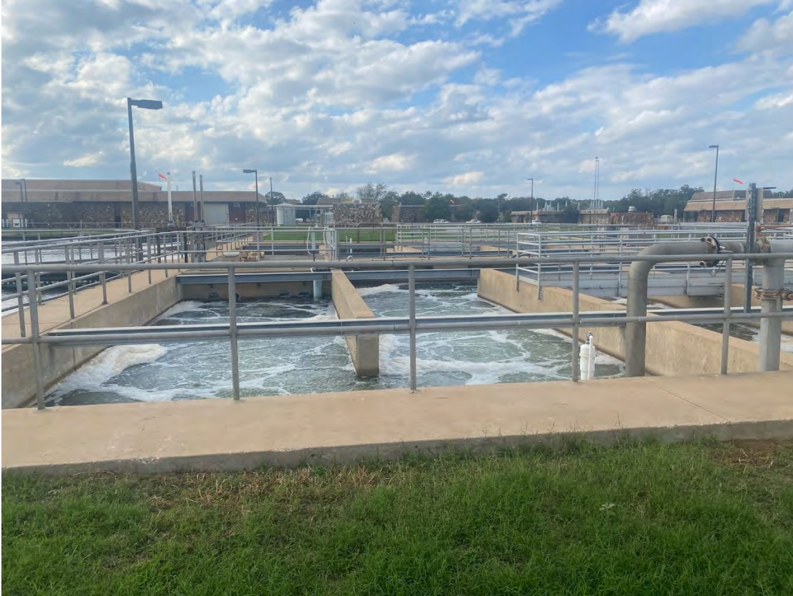
Figure J-9: Chlorine Contact Basin in ASC 1
